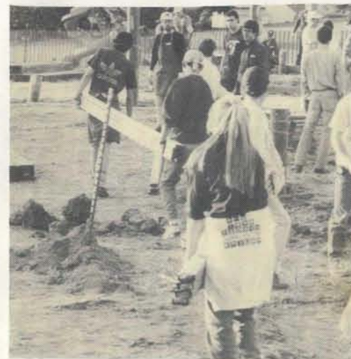
Brothers Scott Bartholomew, Jeff Kendrick and Khrysti Christ bring more lumber to the site.
